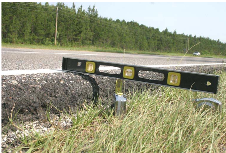
Fig. 3 Shoulder “dropoff” is 5 inches. Many drivers would have trouble if they left the pavement in this area.
