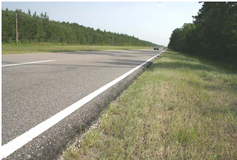
Fig 2 Shoulder dropoff on U.S. Highway 17 near Georgetown, South Carolina. Note the scrape at the pavement edge.
